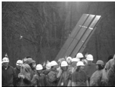
Volunteers help raise Alteris solar panels during the Extreme Home Makeover edition.
