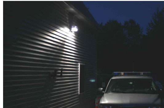
Police station - well-shielded "wall-pack" fixture eliminates glare, directs light downward
