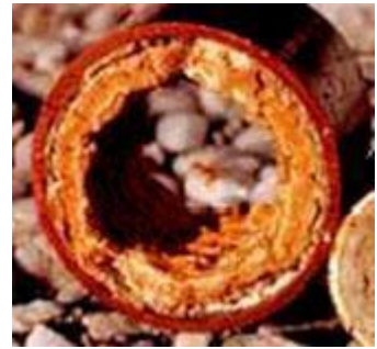
Figure 6: Calcium buildup in a pipe
