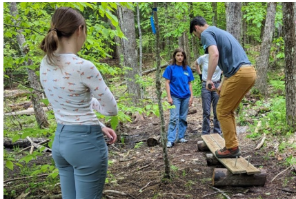
AmeriCorps members build and test a new foot bridge on GMCG's Blue Heron Trail.
