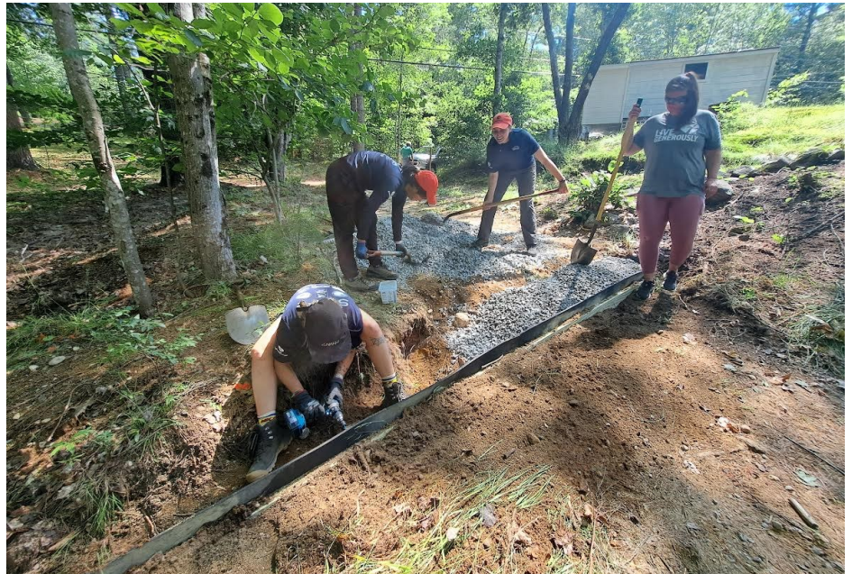
In June, the Friends of the Danforth Ponds (FDOP), a local group of private shoreline homeowners, teamed up with GMCG staff and AmeriCorps to install best management practices (BMPs) such as water bars, infiltration trenches and native blueberry bush plantings to help manage the affects of storm water runoff on the water quality of the Danforth Ponds. The BMPs installed on Middle Danforth Pond are a collaboration including the FDOP, private homeowners and volunteers, GMCG. This project is facilitated with funding provided in part by the U.S. Environmental Protection Agency (EPA) under Section 319 of the Clean Water Act. The funding is administered by the New Hampshire Department of Environmental Services in partnership with the EPA.
